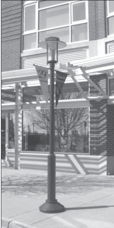
Pedestrian pole lighting with a solid top eliminates light spillover and glare.
