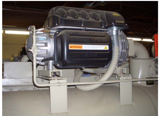
Central Library Chiller (after)
