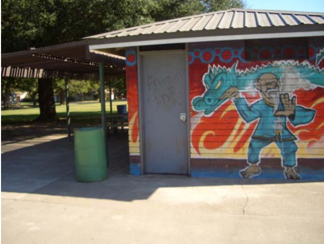
Lawrence Park Restroom Repair (before)
