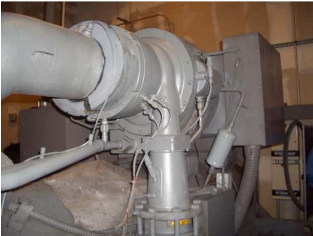
Central Library Chiller (before)
