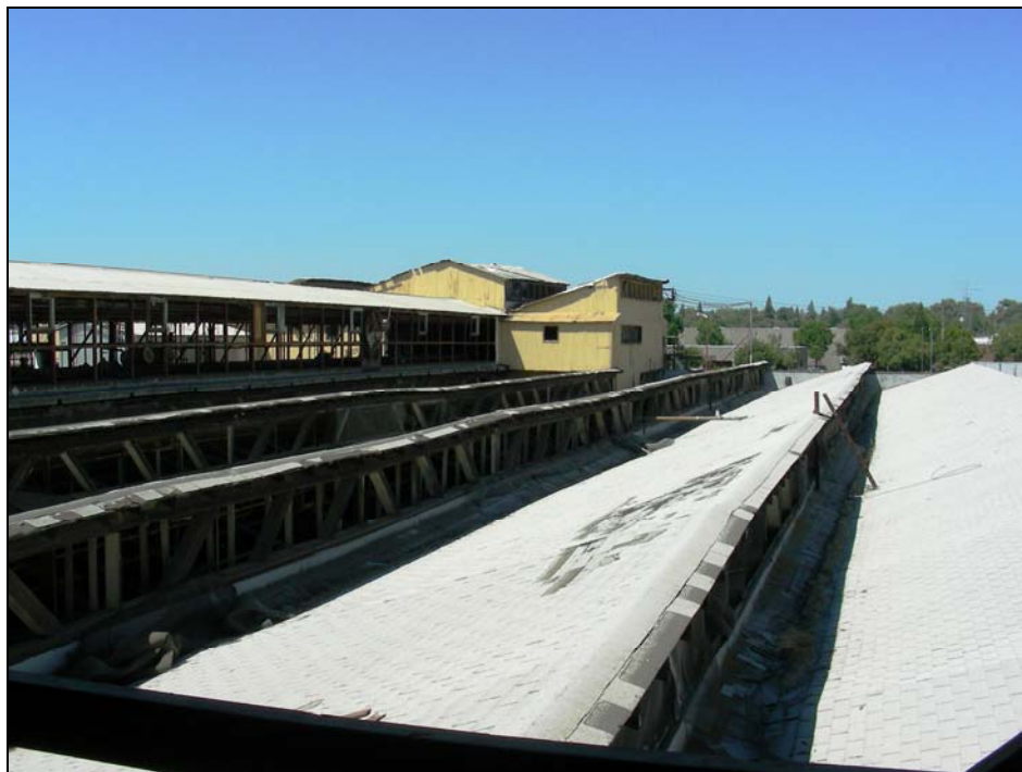
Photograph 17: Building 4, detail of sawtooth roof, can conveyor structure and can loft, camera facing west, 08/29/2006.
