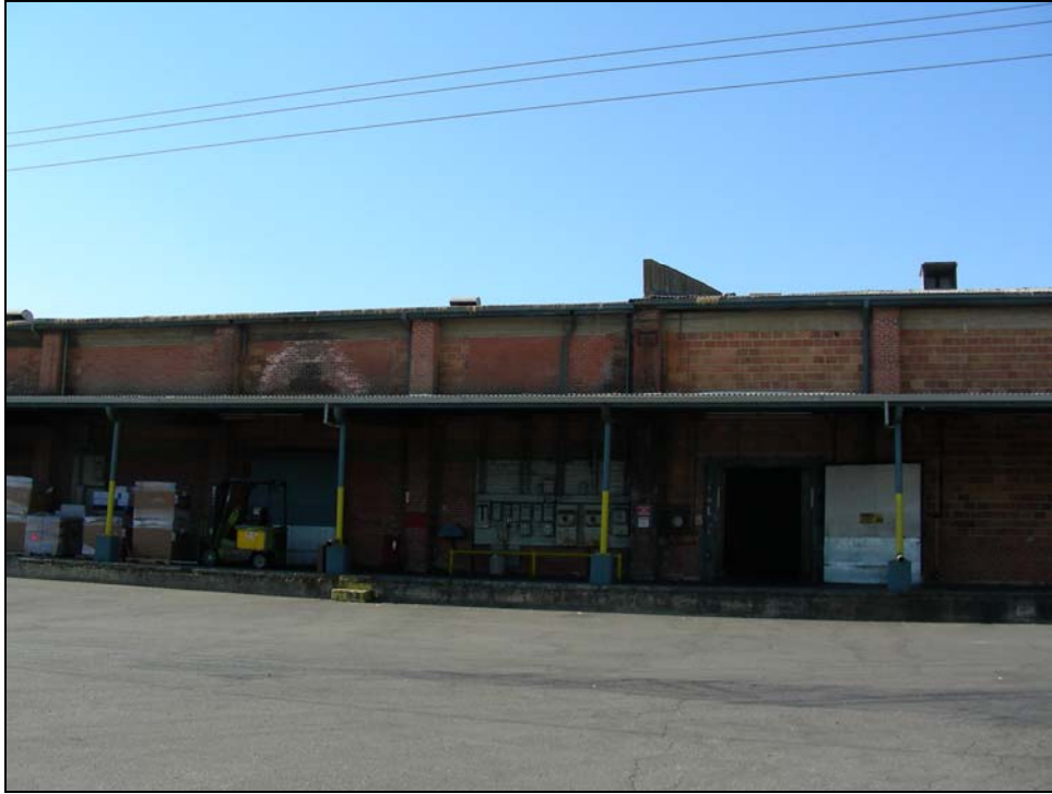
Photograph 6: Building 2, detail showing fire wall between the quick freeze and cold storage sections, camera facing south, 08/29/2006.
