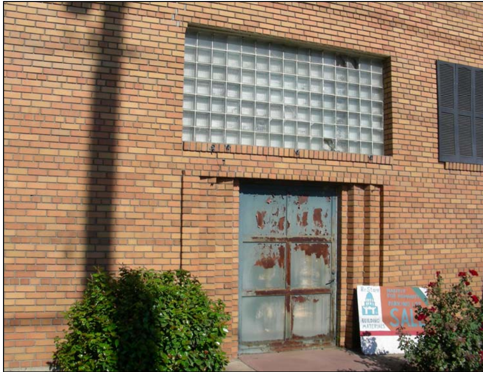
Photograph 4: Building 1, detail of utility door south of main door, camera facing west, 08/29/2006.
