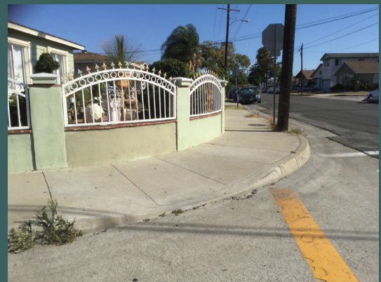
Non-compliant curb ramp
