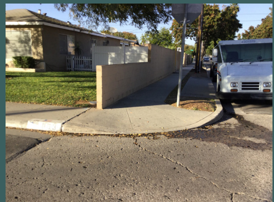
Non-compliant curb ramp
